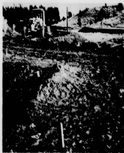
NEW CONSTRUCTION PLUS RAINS caused the field trip some delay and problems in ascending the red butte area on Telephone Hill. A grader made several trips over the road to permit easier travel for Sunlight residents.
