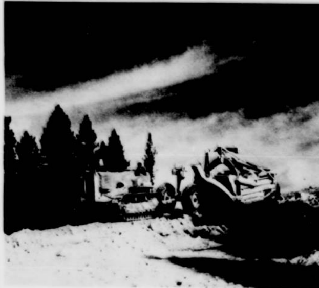
HEAVY EQUIPMENT OPERATORS appear to always be on the skyline. In preparing the new, safe grade, the operators must cut their way along the mountainside, through heavy timber and rocky terrain.
