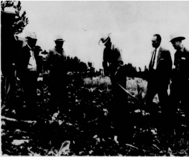
FRANK McCLELLAN, CHAIRMAN OF THE PARK COUNTY BOARD of County Commissioners, turns the symbolic first shovel of earth on the new five-mile Bald Ridge road construction August 10, while a bulldozer waits its turn. Watching McClellan are, left to right, Lynn Bowman, Forest Service engineer; Jim Benson, Grosch Construction employee; P. E. Grosch, contractor; Earl Collins of Pasadena, Calif., and C. E. (Bud) Webster, chairman of the Cody Club road committee. —(Enterprise photos) (See story elsewhere.)
