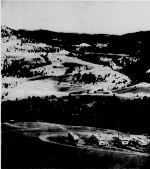
ON THE OTHER SIDE OF THE MOUNTAIN, old and new roads criss-cross as Vern E. Smith, Denver contractor, works on the nine-mile Dead Indian Hill stretch with seven switchbacks that is slated to be finished in October or September. At the right corner of the photo is seen part of Smithville, home of the project workers. —(Enterprise photo)
