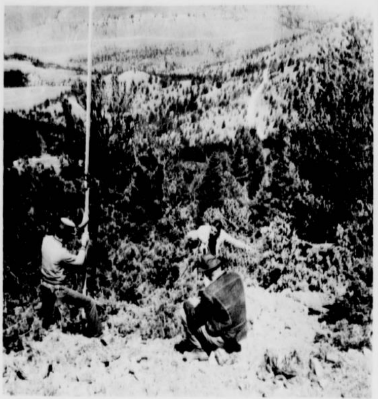
WORK WAS PROCEEDING ON SCHEDULE, despite the highly uneven terrain and strong winds on top of Dead Indian Hill, as Forest Service survey crews laid out the path of the new Cody to Sunlight Basin road. Above, Scott Tucker, Larry Hansel and Mike Smith work at staking levels for the new, wide and less dangerous road. When completed, the road down the slope of Dead Indian Hill to Dead Indian creek will be on an average 6% grade instead of the present 8 to 14% grade. The fifteen or twenty switchbacks curves will be reduced to five, with much wider radius. The entire new road will be twice as wide as the present. Work started out at progress of 2 miles a week, and is now down to about a mile a week due to the difficult timbered slopes. About six weeks is left on the survey job. —(Enterprise photo)
