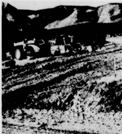
THROUGHOUT THE TRIP the Advisory Committee saw evidence of road construction. This scene shows a new route which will be used on Bald Ridge. —(Enterprise photos)
